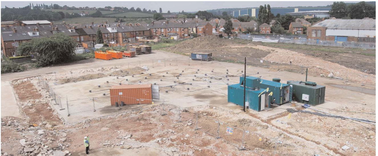
Figure 1: The site of Source Area 1, showing electrode arrays, extraction manifold and equipment locations
